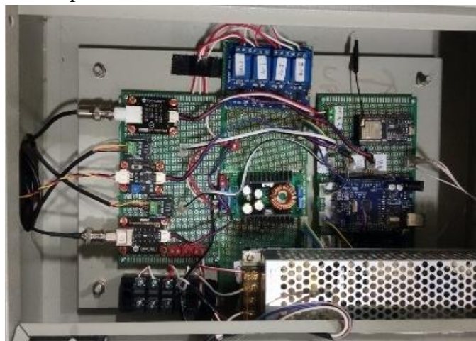
Gambar 3. Panel Kontrol SMARCOS
